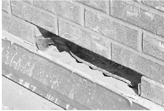
Figure 15-29 Flashing that does not extend through the outside wall face can allow moisture to flow around the front edge of the membrane and back into the wall.
